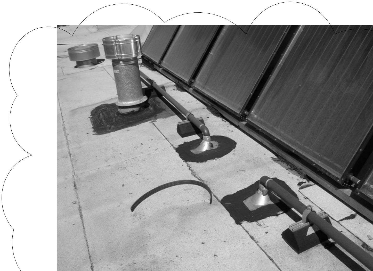
Above Roof Plumbing As-Built Photo
